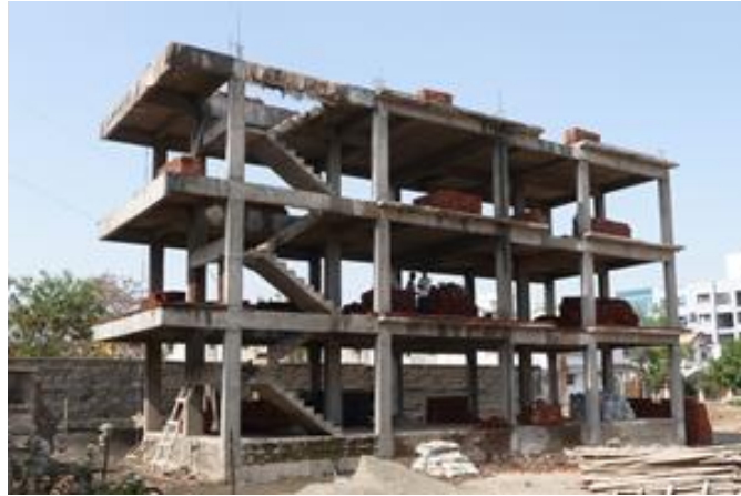
Figure 2. The reinforced concrete floors of this building tie the beams and columns together and force all these parts to move together horizontally during an earthquake.
