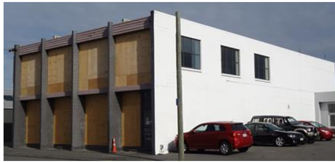
Figure 1. An earthquake damaged building. The strength and stiffness of the long white-colored masonry walls have prevented damaged. A more flexible structural system acting across the building has led to larger movement and damage to the front façade. It is temporarily covered with sheets of plywood.
