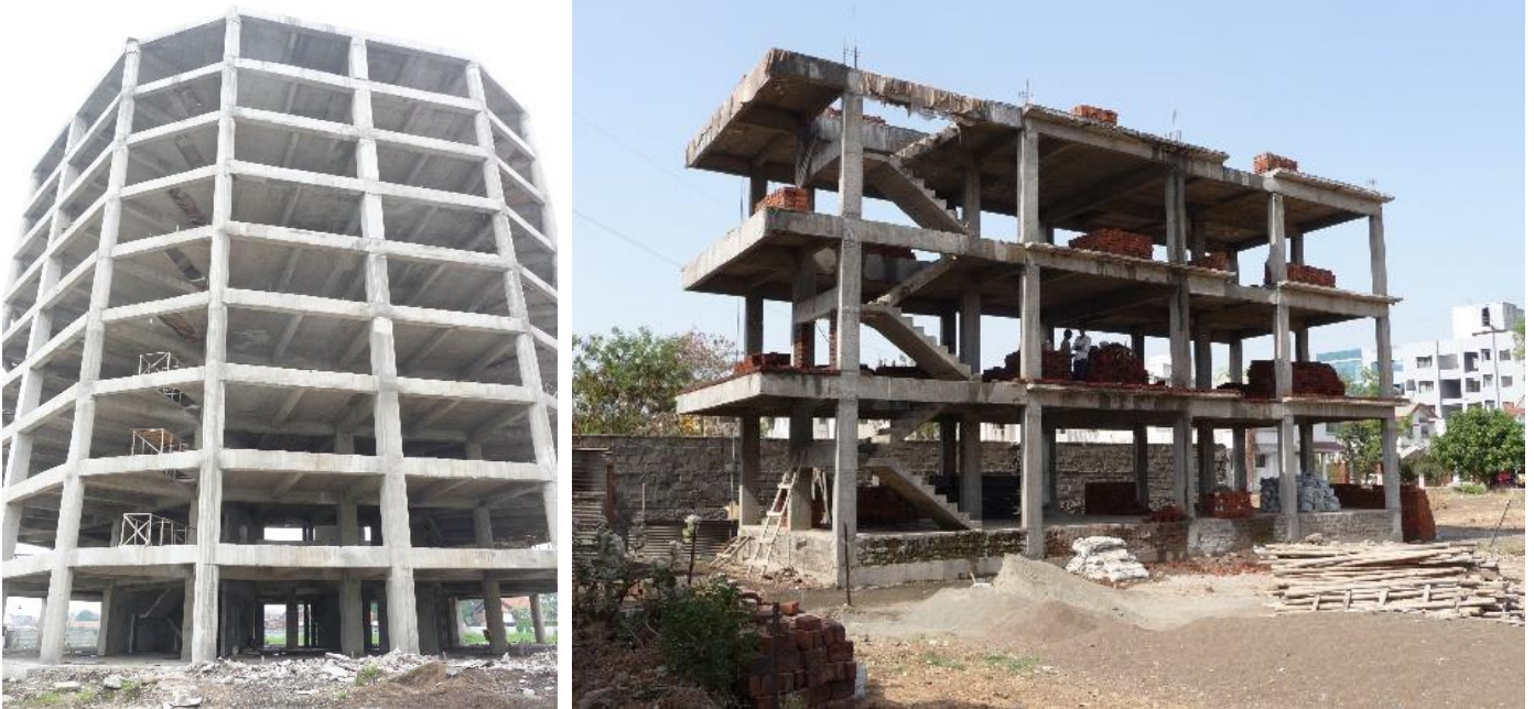
Figure 1. These two buildings resist earthquakes through the strength of their columns and beams. Walls and cladding are yet to be constructed.
