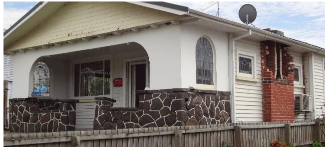
Figure 3. A brick chimney has broken off at roof level and fallen. Most of the remaining chimney is damaged (N. Allaf).
