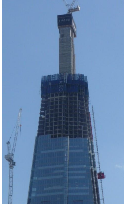
Figure 3. An example of a reinforced concrete core in a building under construction.
