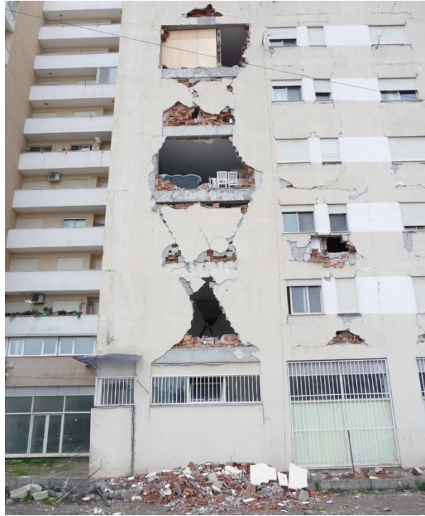
Figure 2. An example of an earthquake damaged building where the infill walls have not been carefully designed to allow for forces and movements during an earthquake.
