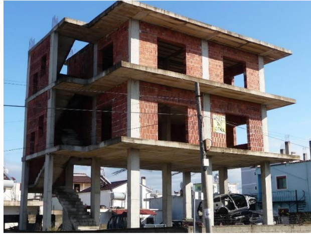
Figure 5. A typical soft story building where the ground floor is the weakest.
