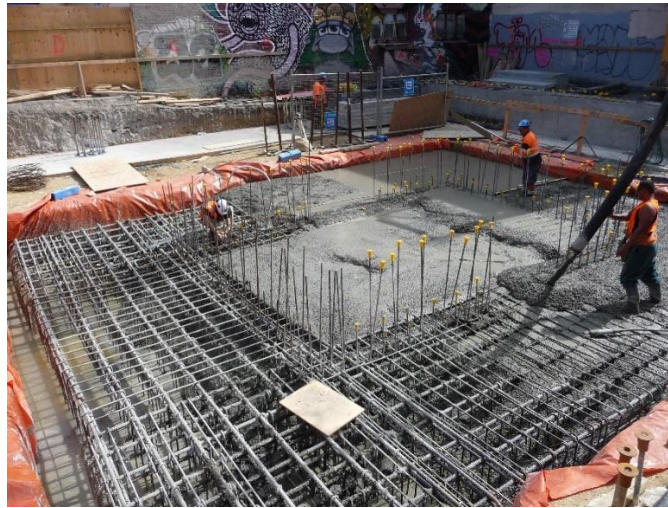
Figure 3. The foundations of a building under construction. Engineers have followed codes to determine the amount of reinforcing steel and its correct location.
