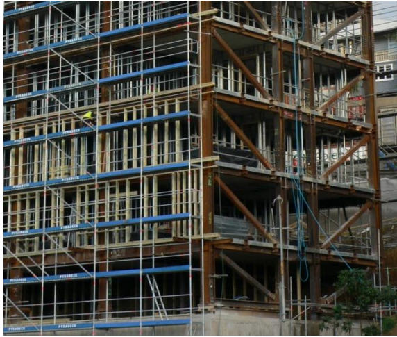
Figure 3. Steel braced frames resist earthquake forces acting across the building. Steel moment frames provide strength along the building.
