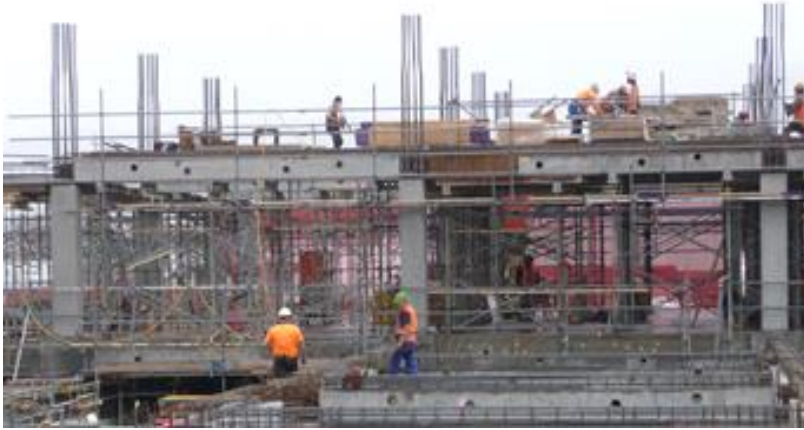
Figure 3. An engineer needs to regularly visit construction sites like this to ensure construction is in accordance with the plans and specifications.
