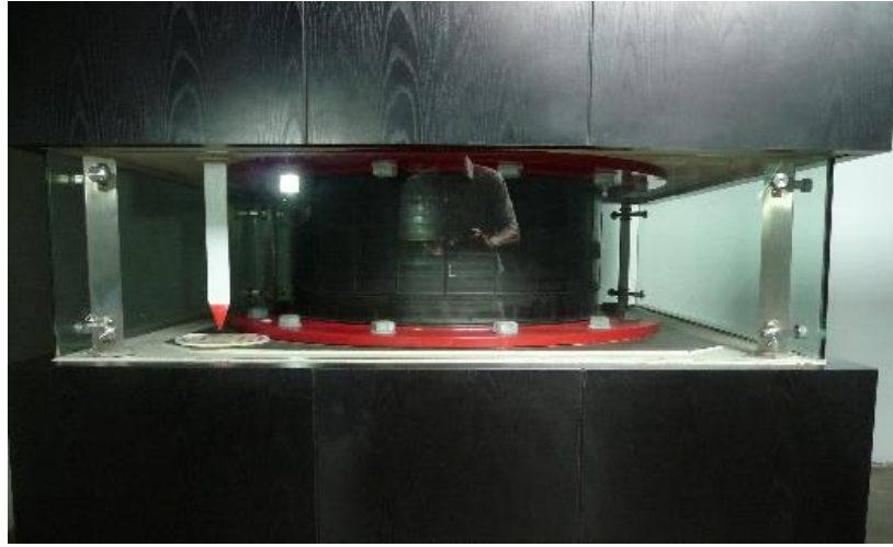
Figure 4. A circular rubber bearing containing many thin steel plates is located between the bottom of every column and its foundation to isolate the building from horizontal earthquake shaking.
