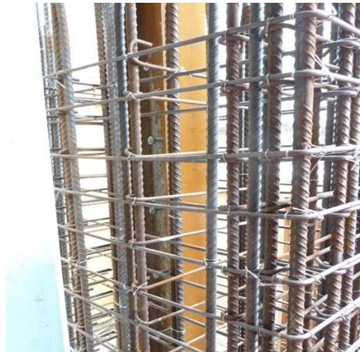
Figure 3. Column reinforcement is visible before the concrete is cast. The reinforcement consists of vertical bars that resist bending, and horizontal ties that stop the column concrete from disintegrating and dislodging.
