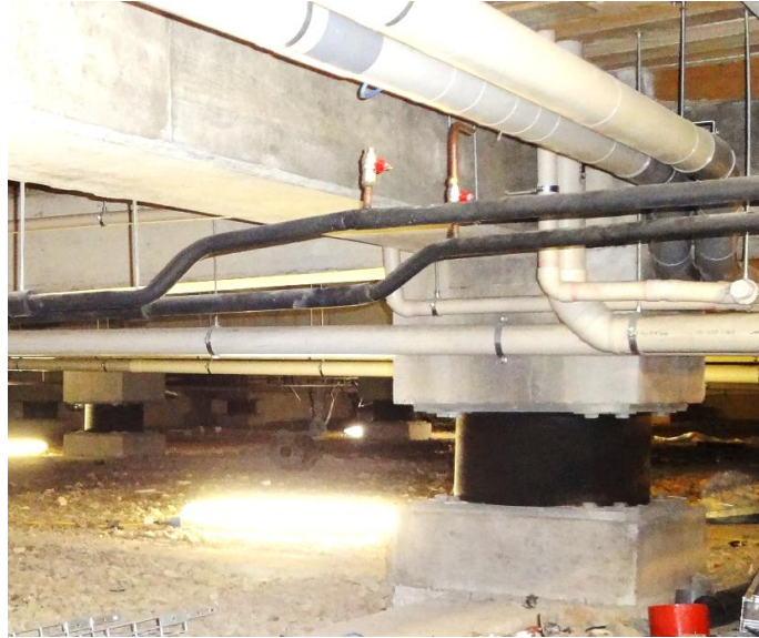
Figure 2. Two black and cylindrical isolation bearings under a building. Each bearing is bolted to a concrete base attached to the foundation and the base of a column that rises up the building.
