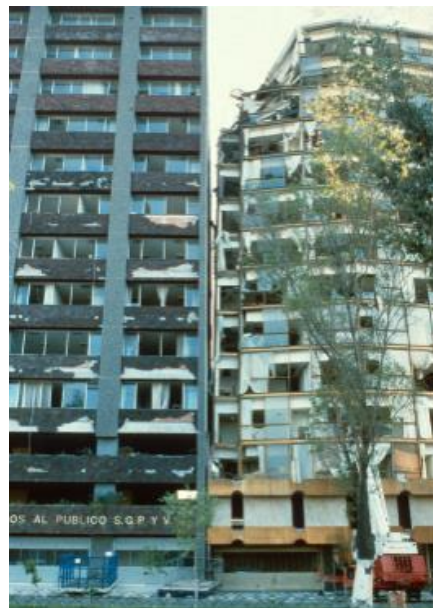
Figure 2. Two buildings have pounded each other with one far more seriously damaged than the other.
