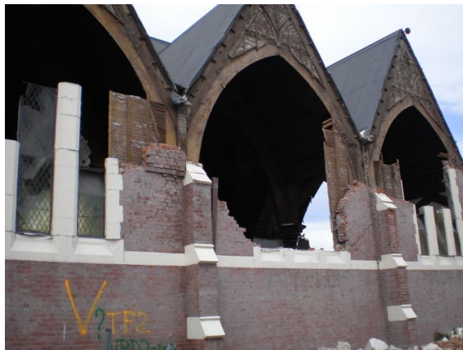
Figure 4. An earthquake has destroyed most of the brick cladding and glazing of this building.
