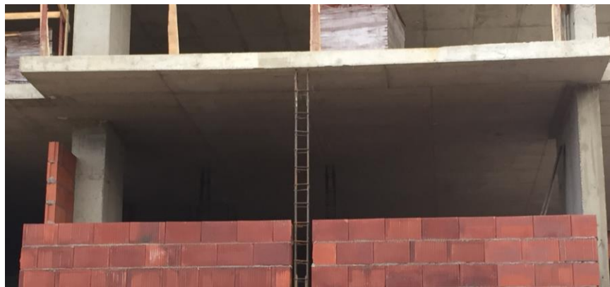
Figure 4. An example of an intermediate column to stabilize a masonry wall (S.Brzev).
