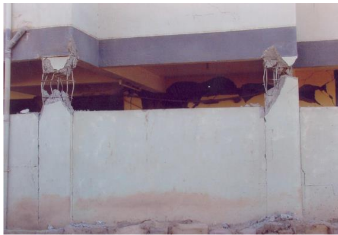
Figure 4. Earthquake-damaged short columns.
